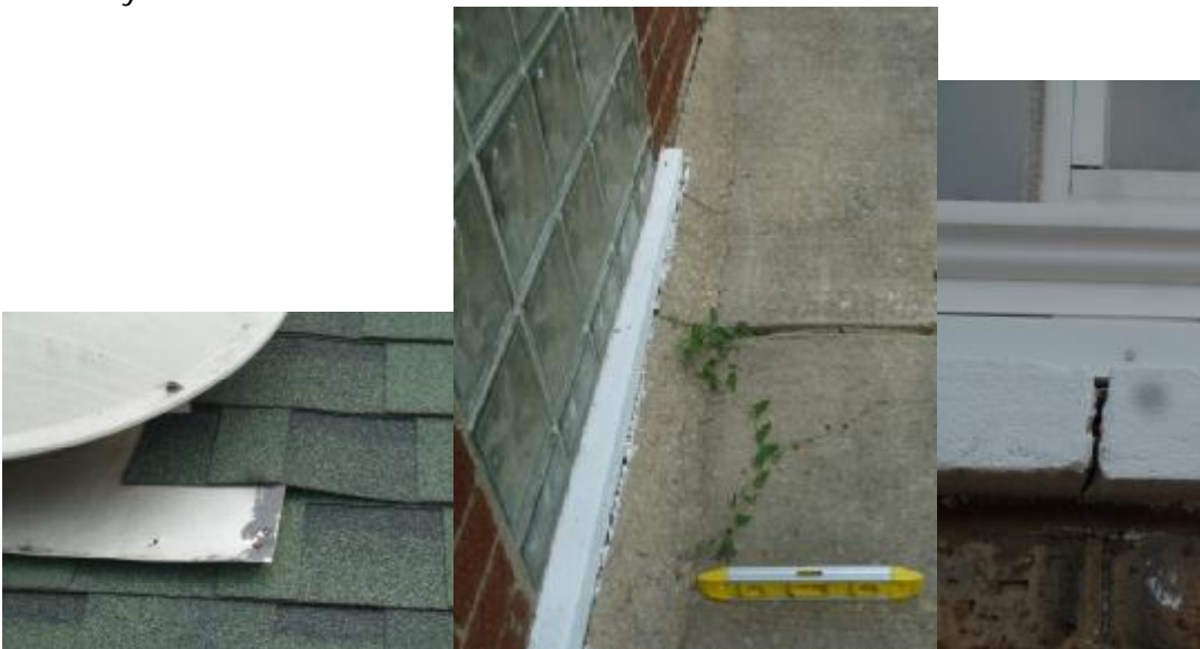
loose nail, powered fan; concrete sloping toward house, cracks at cement patching attempts, south wall; cracked stone sill at N bedroom window, likely an indication of a foundation wall below
