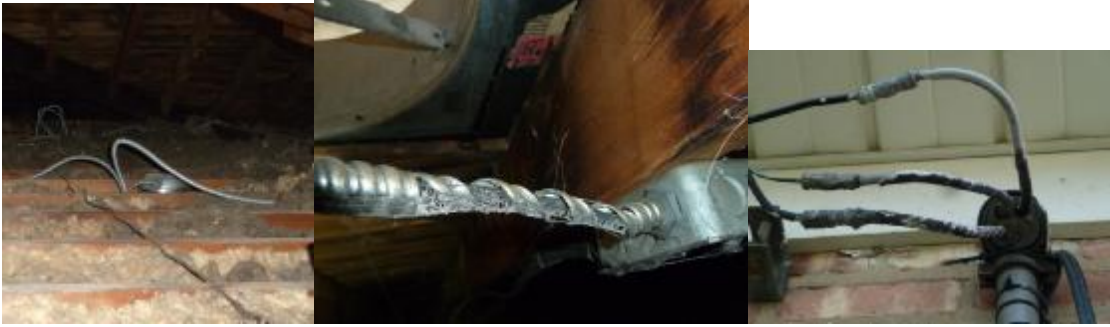
Loose cables, attic, incl. near fan; frayed insulation at elec. service wires
