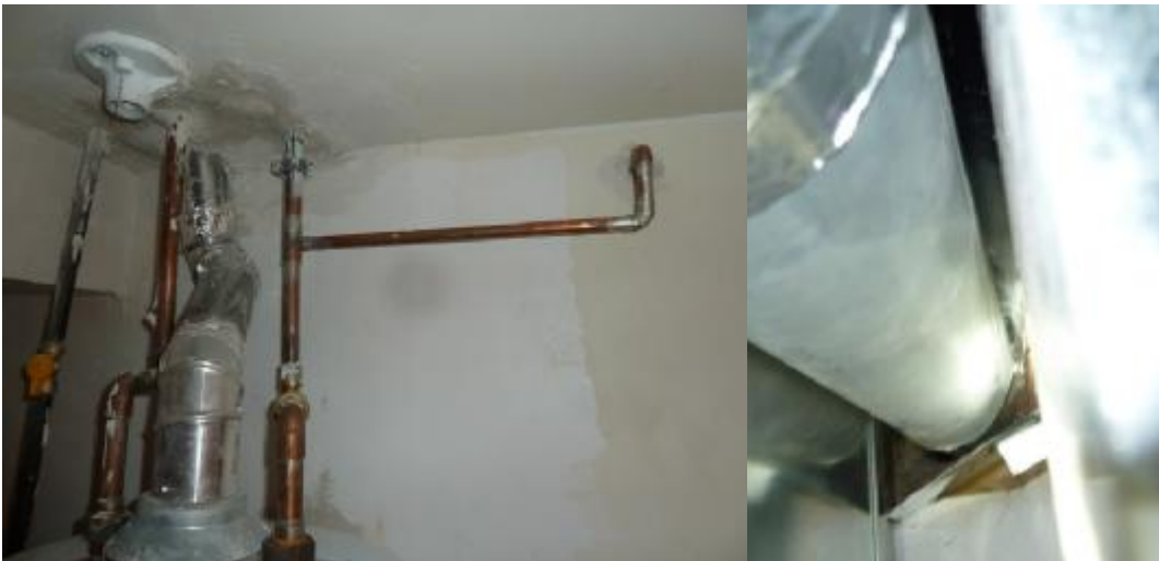
Water heater exhaust vent installed poorly, improperly concealed, backdrafts; note lack of shutoff valve for rear hose faucet piping
