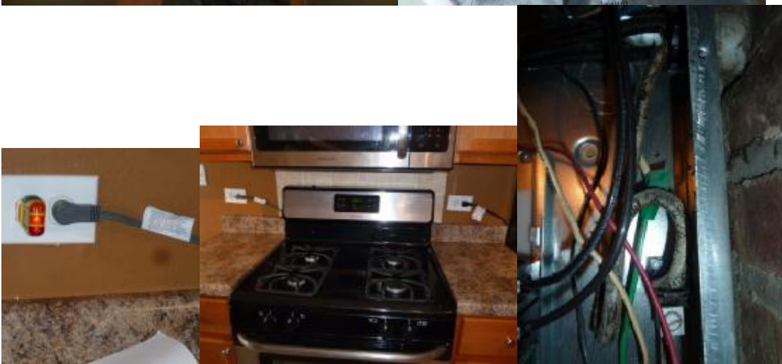
Reversed polarity outlet, standard non-GFCI outlets not provided for appl's, GFCI outlets not completed at counter. Spliced ground wire, main panel
