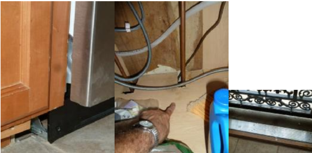
Gap at DW; small leak under sink; gap under side door
